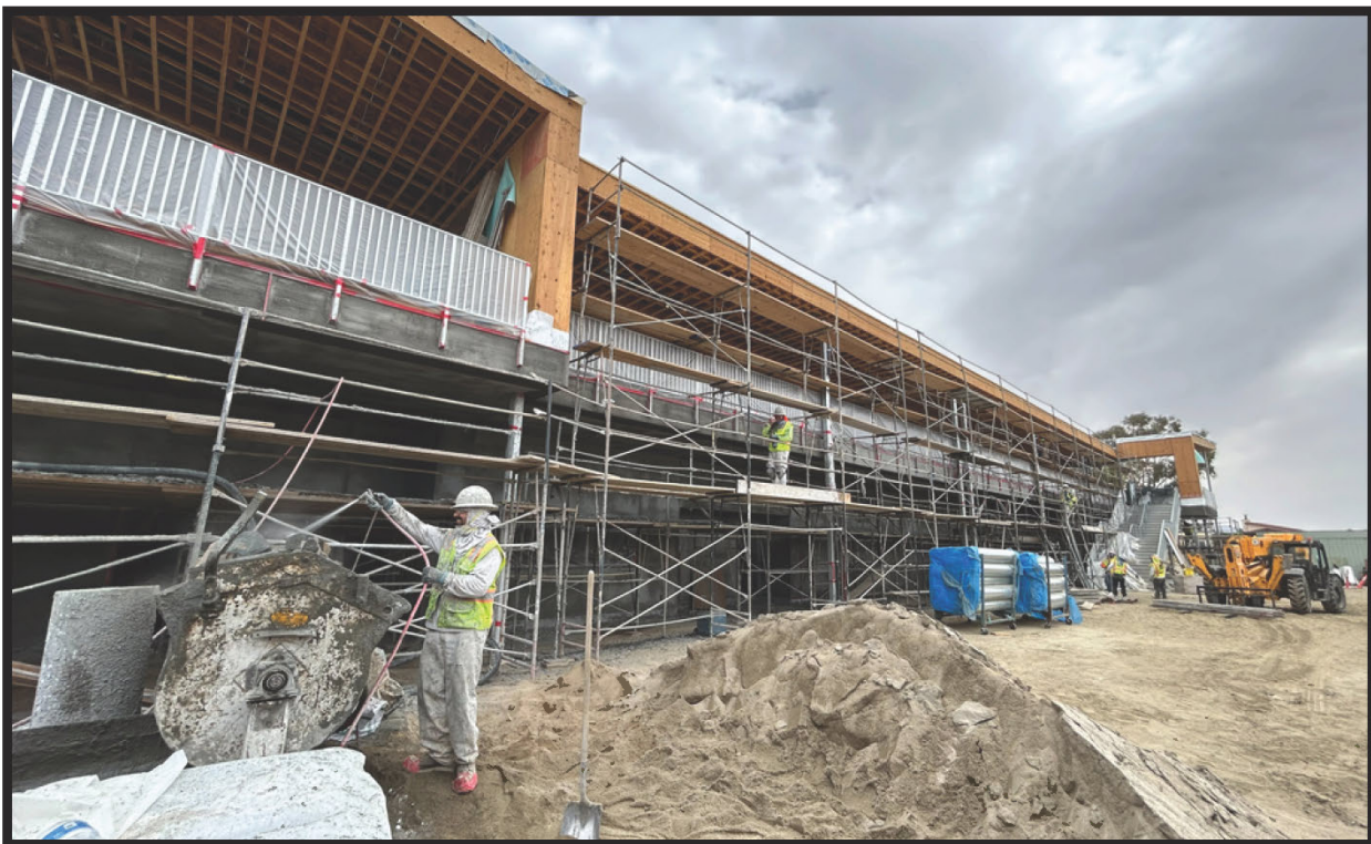
Journeyman, Julian Godinez working on cement pump at Landau Elementary School in the City of Cathedral
